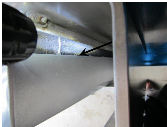
Fig. 6.2-6: Little water leakage on the bolt side
