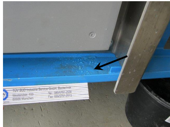
Fig. 6.3-4: Little water leakage on the bolt side
