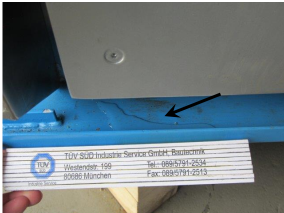
Fig. 6.3-3: Little water leakage on the hinge side, forms a small trickle
