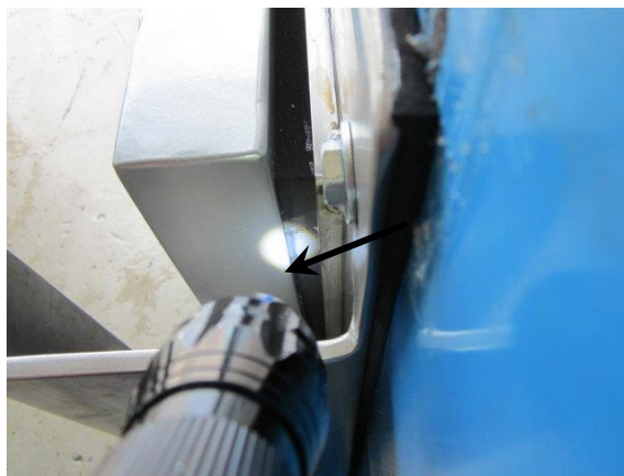
Fig. 6.2-5: Water leakage on the bolt side in the top right-hand corner (mitre joint not clean)
